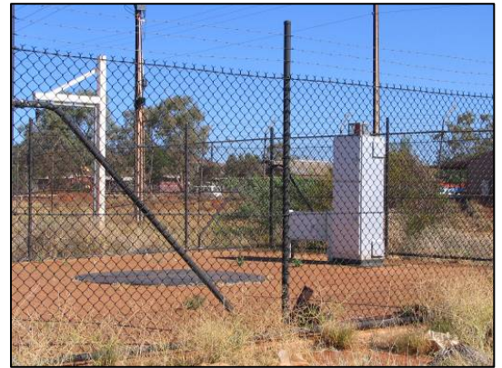
Stand Pipe & Sewer Pump Station
