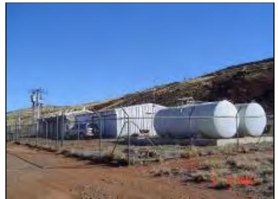
Power generation compound
