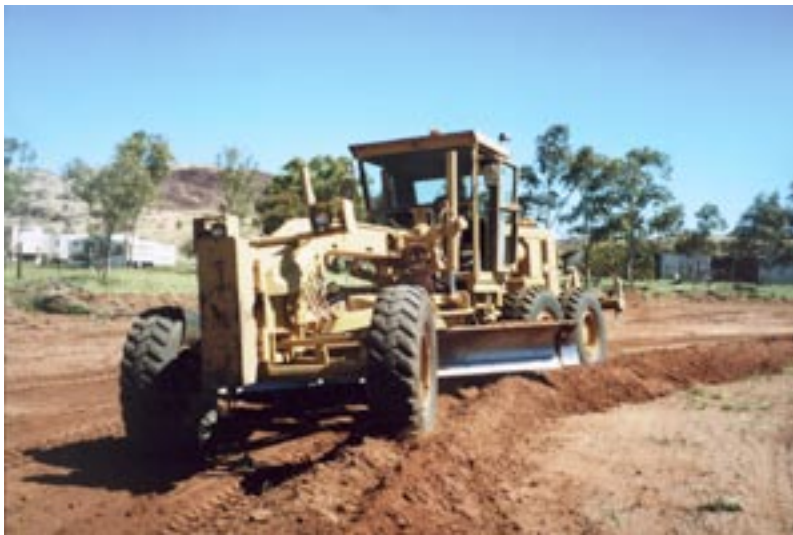
7. The wheels of the road grader are used to roll and compact the bank during construction [March 2001].
