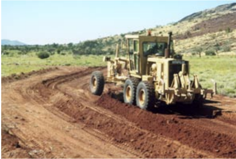
5. View of ponding bank construction at Kalka. The grass has been cleared away and soil is being turned in from the top side to form the bank [March 2001].
