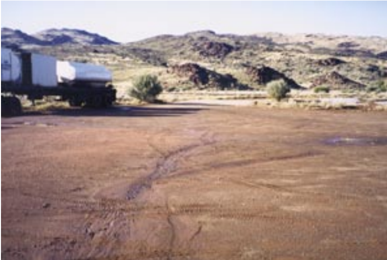
13. Storm water collects on open compacted areas around communities and if left unchecked, begins to flow and cause erosion [October 2001].
