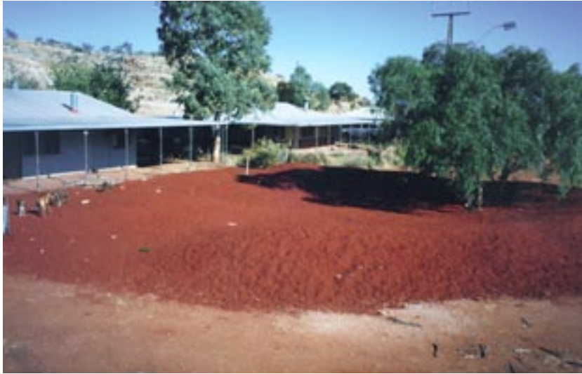
5. This mound system was built in the front yard of a house at Pipalyatjara. It was constructed around two mature pepper corn trees and collects storm water from the roof and yard [June 2001].
