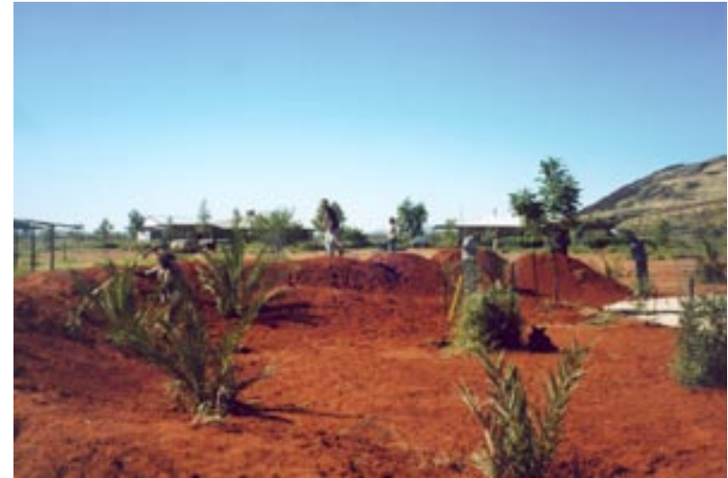
18. View of part of the mound system which surrounds the office at Kalka. This area collects a large portion of the storm water harvested from the roof of the office [April 2001].
