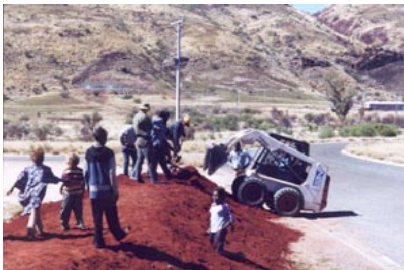
3. A bobcat is being used to shape the outside slope of the first mound at Pipalyatjara. School children were a great help shaping the mounds [October 2000].
