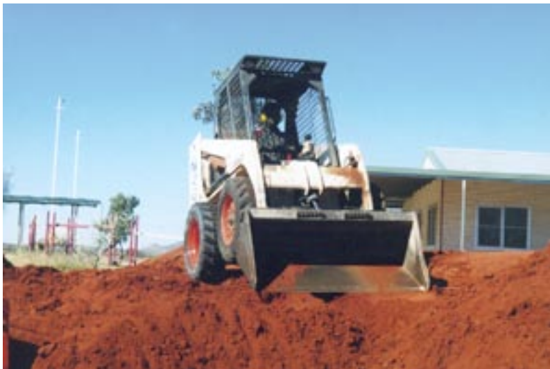
15. View of a bobcat being used to shape and level the top of the Amphitheatre at Pipalyatjara [May 2001].
