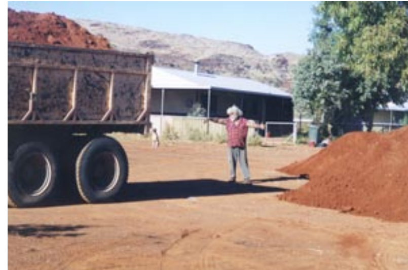
10. Care should be exercised at all times and truck drivers should be given clear directions when soil is being tipped from large trucks. Mounds are easier to shape when soil is tipped in the correct location [August 2001].
